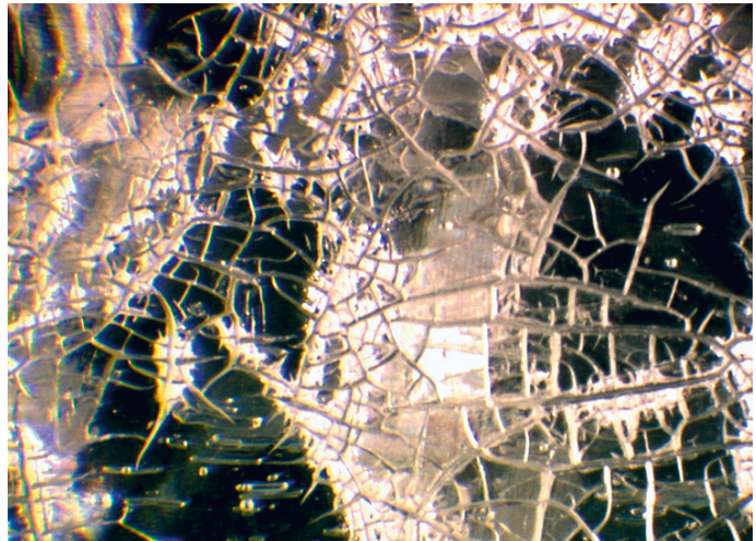
Figure 11, GF-UP sheet, transparent (M = 20, AL + DL). The cracks (hair cracks) in the sample surface developed after 5000 hours of weathering in a Xenon tester 1200 CPS. The crack depth is no deeper than about 35 µm. During recording, a low level of transmitted light has been combined with incident light.
